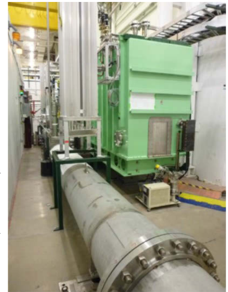
Test bunker containing the FRIB prototype \beta_0=0.085 cryomodule and the prototype cryogenic distribution line.
