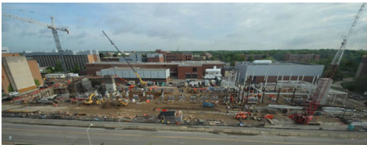
Site of FRIB civil construction. Construction of the underground accelerator tunnel is completed.
