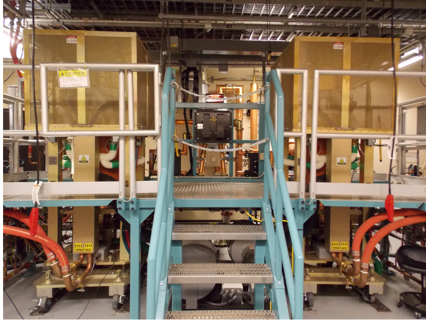
Figure 1.5: The new LANSCE 201RF MHz Diacrode FPA for DTL Modules 2-4.
