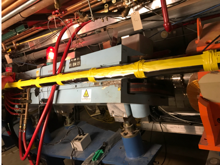
Figure 5.18: Mu-metal shielding installed along the entire length of WNR beam pipe effecting by the RIBM01 residual magnetic field.
