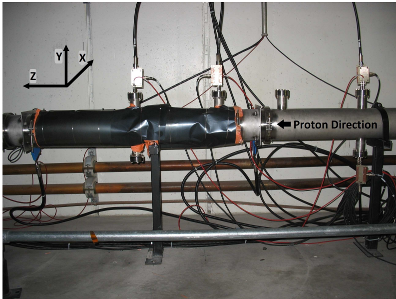
Figure 22: The TiN coated section of beam pipe was wrapped in mu metal in order to compare signals with and without magnetic shielding.
