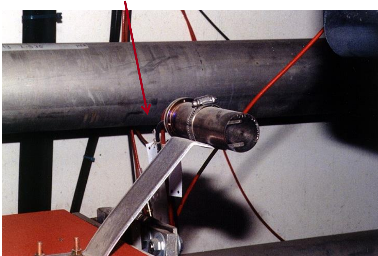
PMT loss monitors
