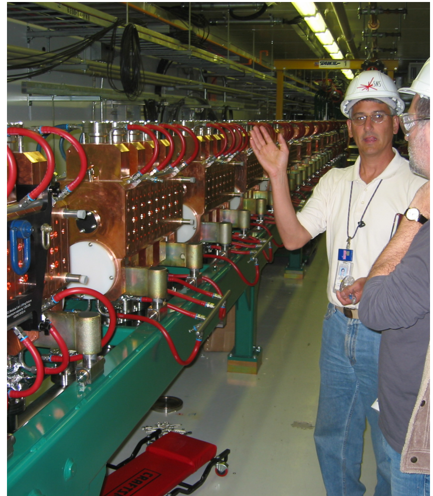
SNS CCDTL tanks installed in tunnel
